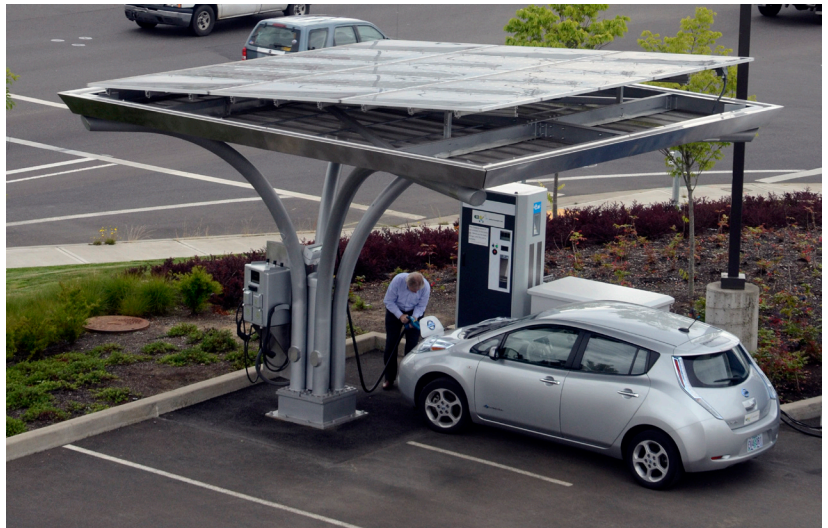
EV4 Oregon's first installation is located in Tualatin, at Powin Energy's main offices, and is a great demonstration of the technology's benefits.
