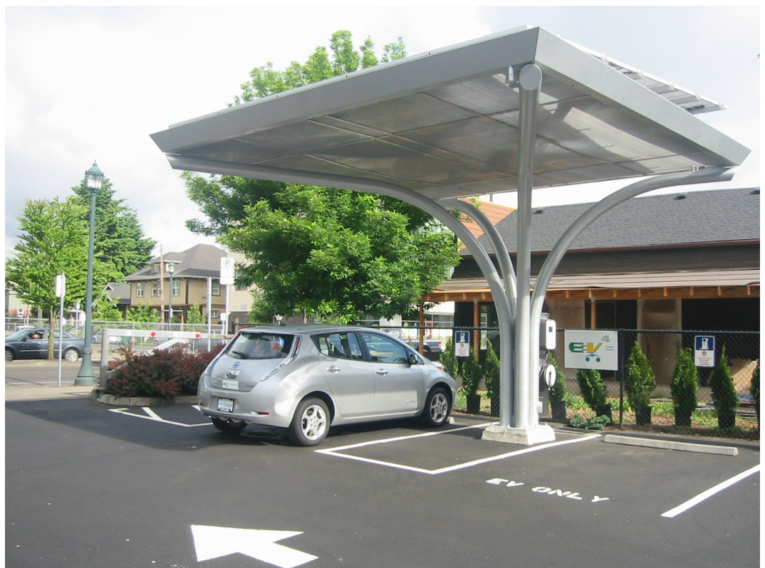
EV4 Oregon's first installed ETM™ station with a solar canopy, located in NE Portland.
